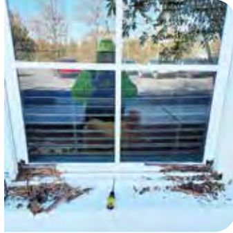
Window in need of repair, Deerfield Golf Course
