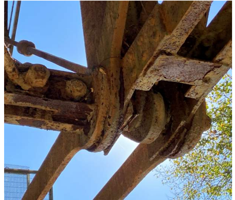
Corroded Truss Connections
