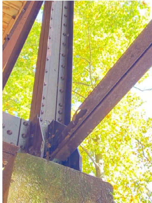
Section Loss on Truss Members
