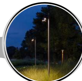
▲ PEDESTRIAN LIGHT POLE
